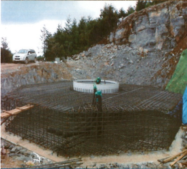
Wind Farm - Taebaek 18MW
